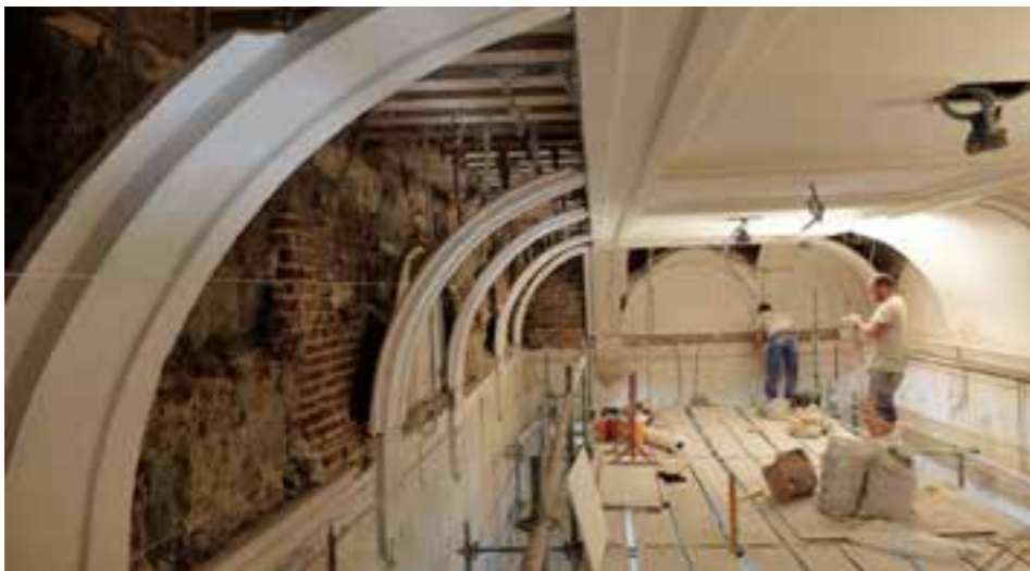
1. Narthex of the Convent of the Comendadoras of Santiago, Madrid, before the restoration works 2. Restoration works in the narthex of the Convent of the Comendadoras of Santiago, Madrid 3. Patio of Moradillo in the Convent of the Comendadoras of Santiago, Madrid, after its restoration.
