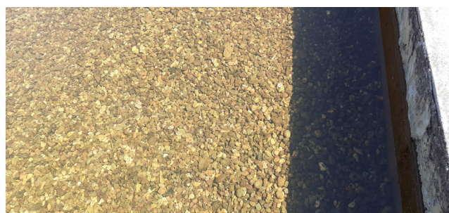
Figure 2. Gravel filter with presence of mud on the surface. a) week 3; b) week 10.
