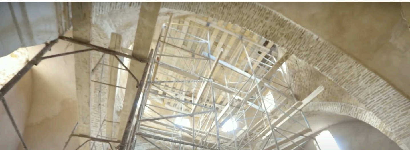
Figure 2: Screenshot from a video of the renovation work of the Hammam El Bey, National Federation of Tunisian Communes (2020). [4]
