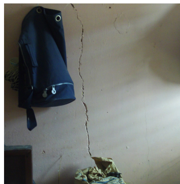
c) Cracks or fissures (Level III)
