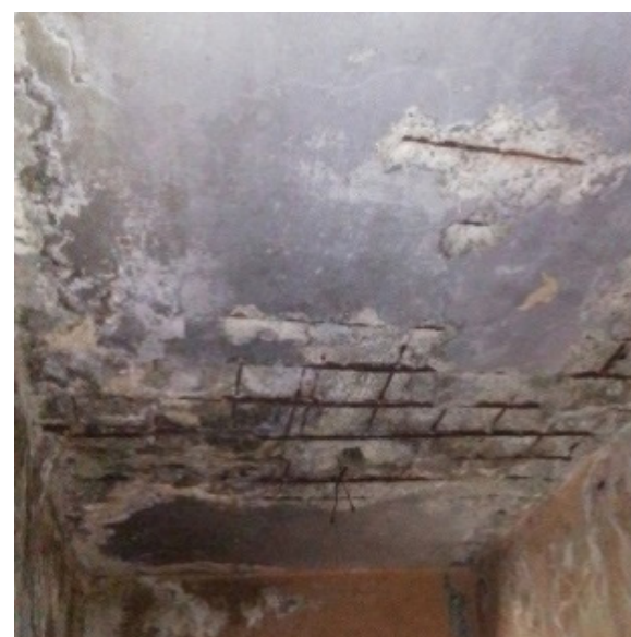
d) Mechanisms of concrete decomposition and Corrosion of armor (Level III)
