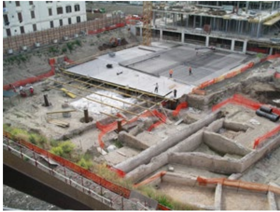
[Fig. 11] Roma, excavations in the district of Testaccio, construction of the new market on the remains of ancient stores. Author's photograph, 2004.
