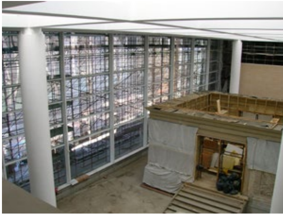
[Fig. 8] Rome, the Ara Pacis Augustae during the construction of the roof designed by Richard Meier. Author's photograph, 2006.
