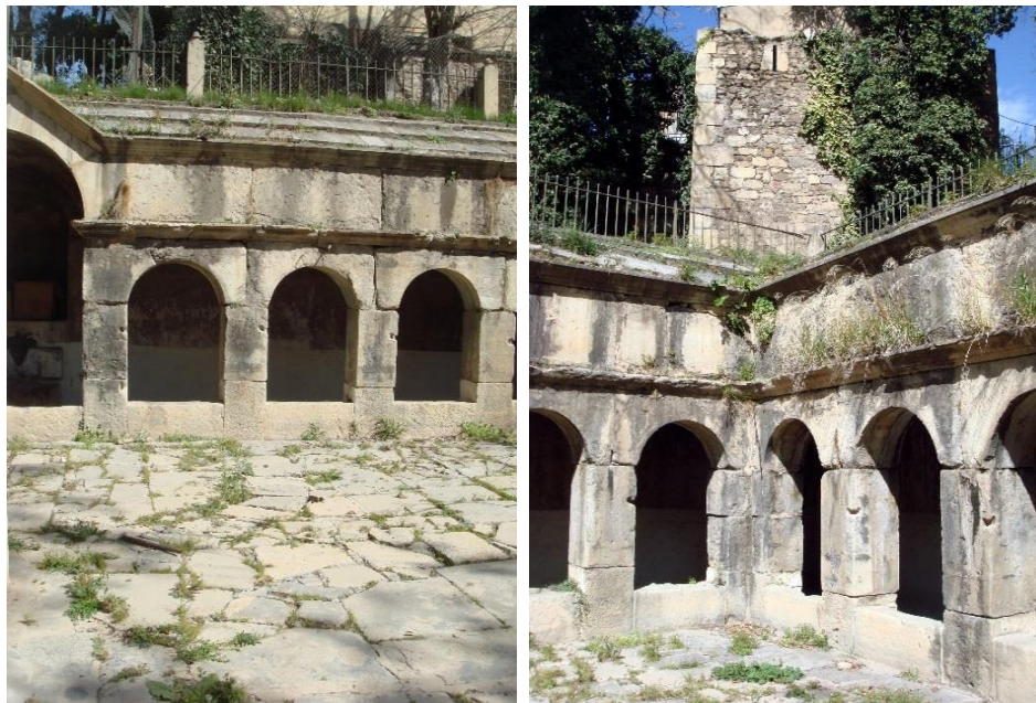
Figure 4. View of the crown of arcades and its curved central opening on the East side of the building. © MAHDADI, N. 2020.
