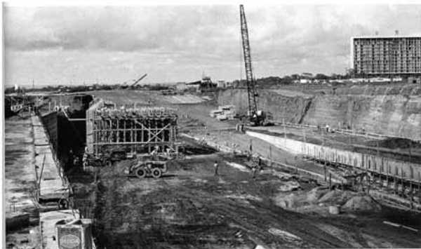
Figure 4. Construction of the foundations of the ministry buildings in Brasília (DF Public Archives)
