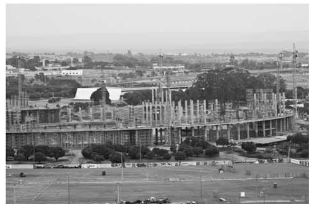
Figure 8. Picture from the recently finished sports arena in Brasilia during construction stage
