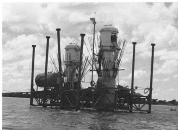
Figure 5. Example of pressurized drilled caisson platform and work site over a river in Brazil
