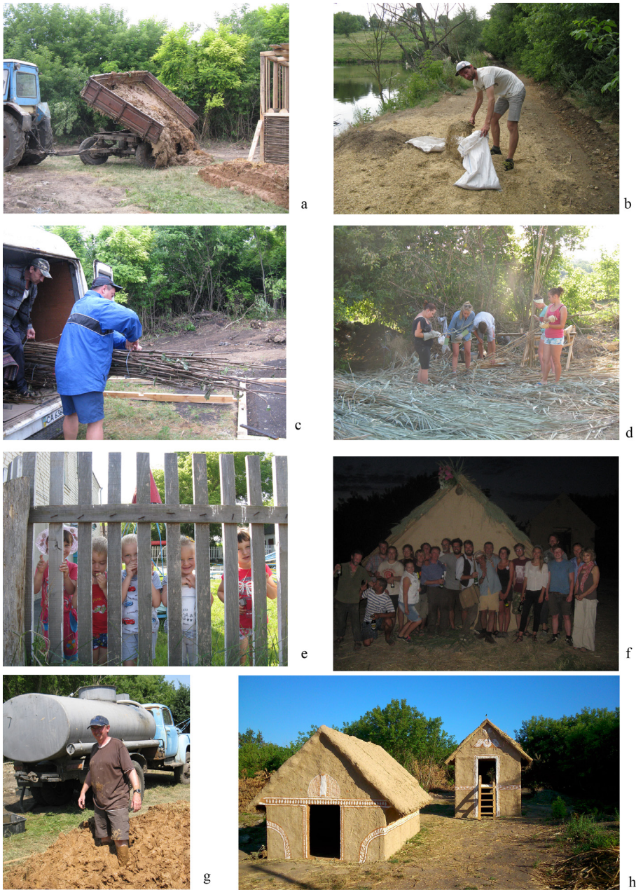
Fig. 8. (a) The delivery of the clay; (b) Vlad Litkevych collecting chaff; (c) Collecting hazel withies; (d) Sorting reeds for roof thatching; (e) Village children quietly observing the building from the kindergarten; (f) The party after completion of the two houses; (g) The project manager gets his boots dirty mixing clay; (h) The two completed experimental houses (B. Gaydarska).
