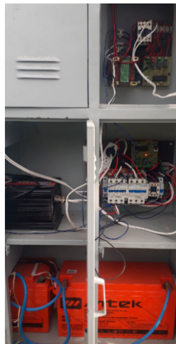
Fig. 8. Complete electrical system implemented for the experimental test. Source: Authors.
