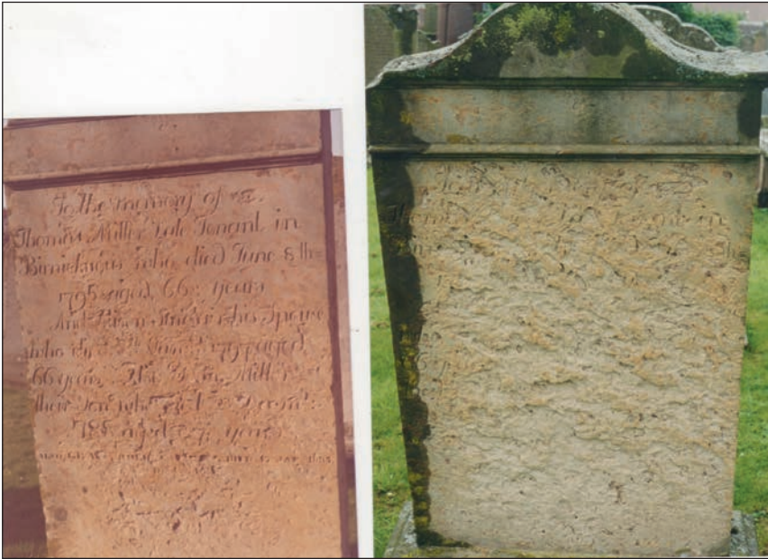
Grave of Thomas Miller (1729-1795) & Alison Sinclair (1730-1797) showing erosion and loss of text.
