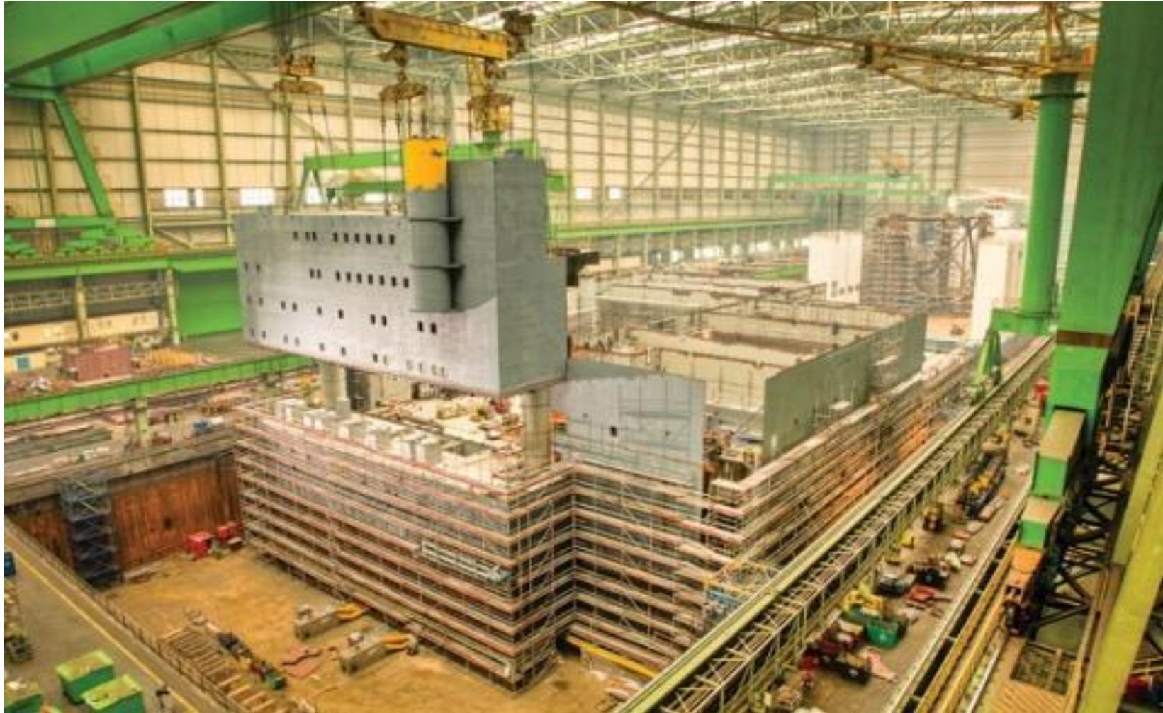
At dockyards near the North Sea port of Rostock, Germany, Siemens is building a massive platform that will house equipment for managing power from wind farms far offshore.
