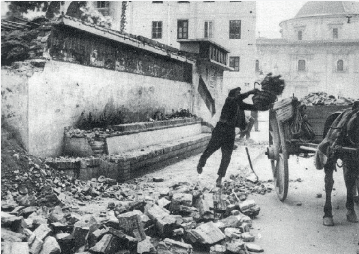
Process of dismantling of the shelter in the garden of the Palau de la Generalitat, Plaça de la Mare de Déu. Photograph: Unknown author (Valencia, 1945).
