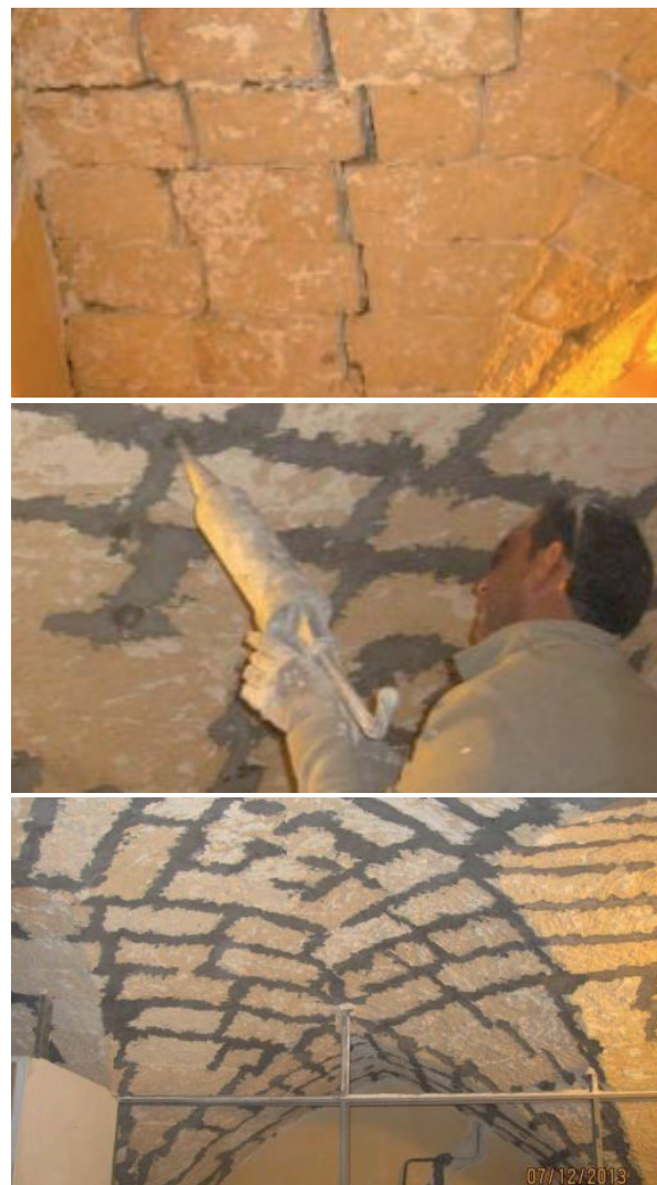
Figure 17. Injection of mortar at the vault intrados. a) before strengthening b) strengthening c) after strengthening.
