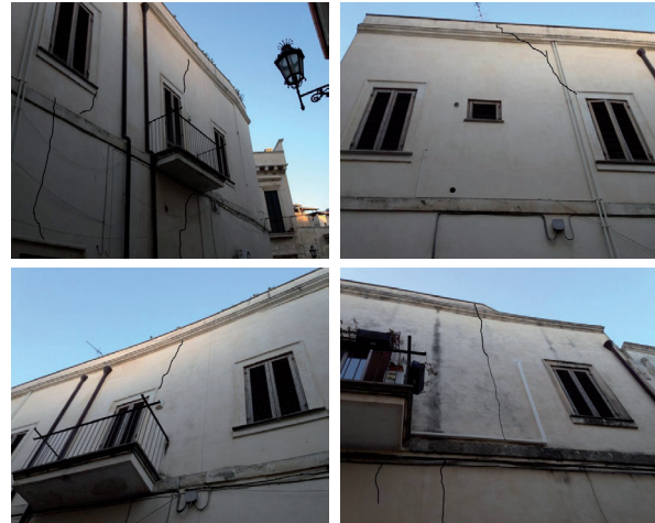
Figure 13. Cracks on the external walls.
