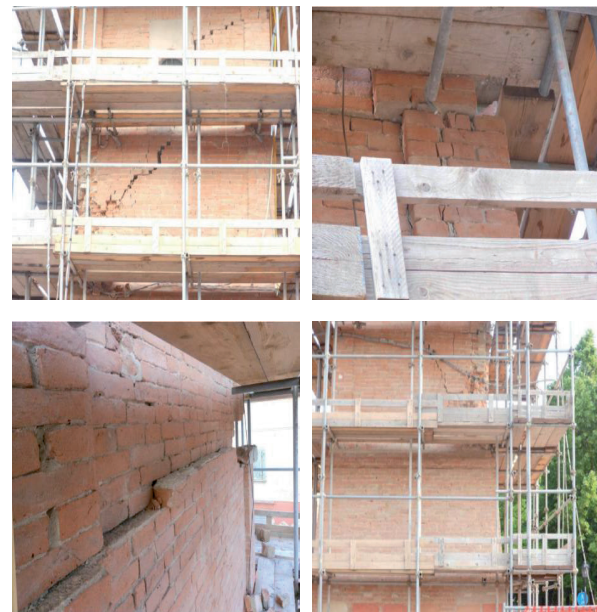
Figure 8. Main damage resulting from the May 2012 earthquake in Emilia: a) diagonal crack (west side), b) dislocation A (20cm), c) dislocation B (6cm), d) cracks (north side).
