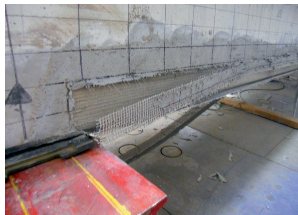
Figure 8. Failure of the cementitious composite strengthening in the beam TTsf.
