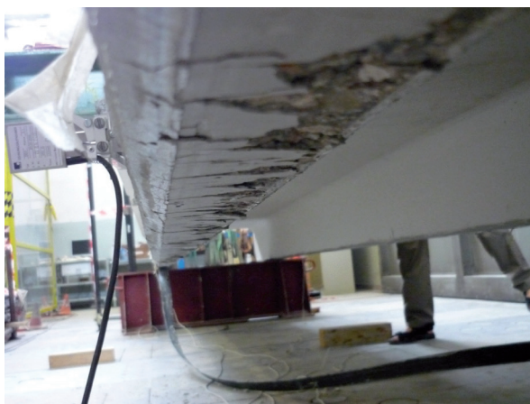
Figure 6. Detail of the TTcl beam after the test.
