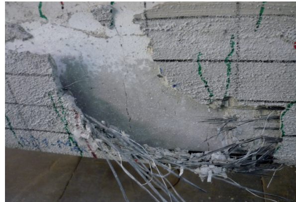
Figure 7. Detail of the fibres after the concrete cover removal.
