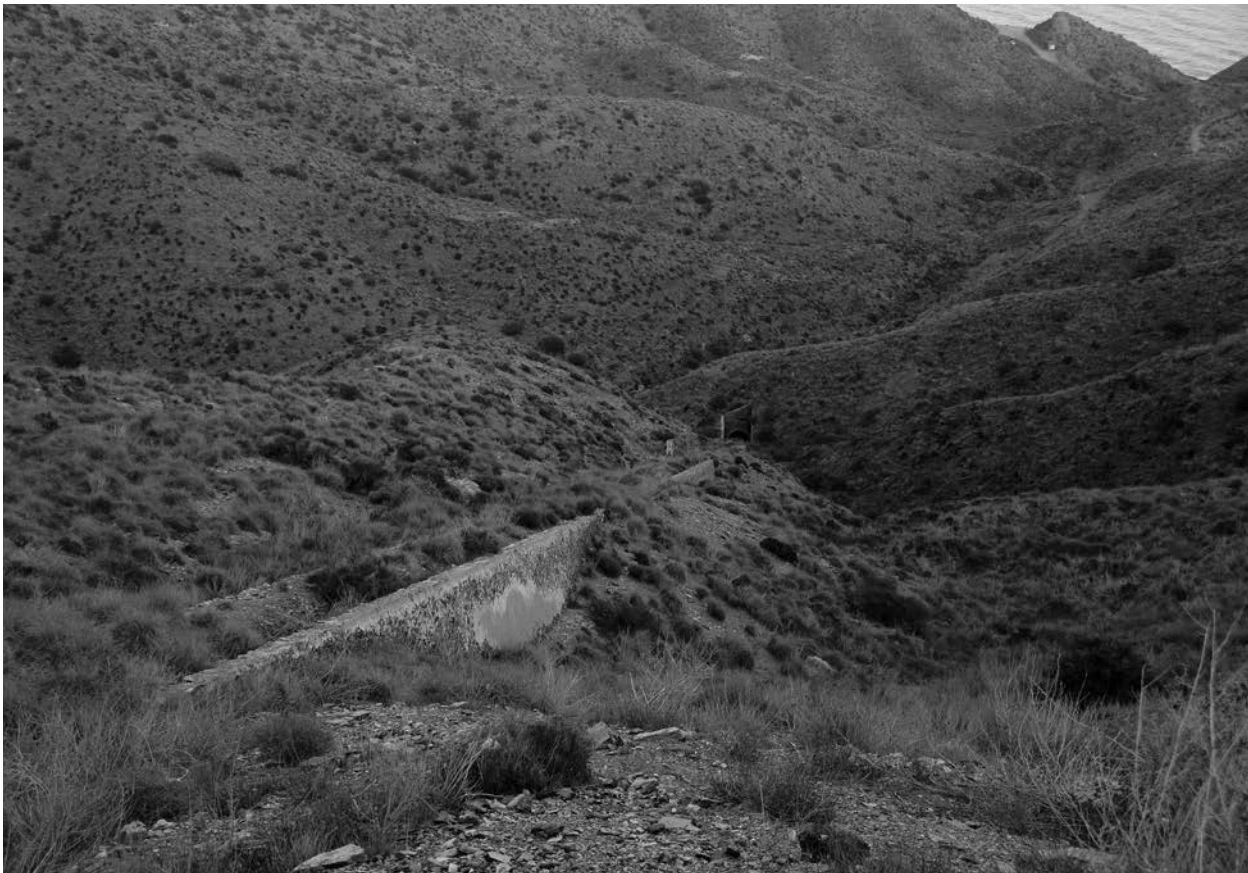
Figura 12. Plano inclinado vertiente marítima. Figure 12. Inclined plane on the side facing the sea.
