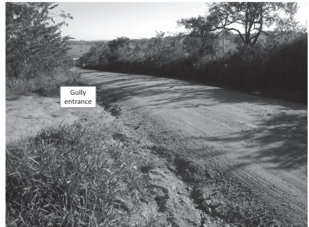
Figure 3. Cravo Stream Gully entrance, Nazareno, Minas Gerais (Brazil). The compacted road that does not have a proper drainage system can be seen. Source: The authors.
