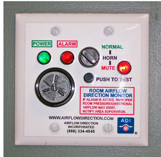
Fig. 4. Airborne Infection Isolation (AII) room pressure monitor.
