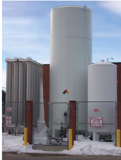
Fig. 5. Liquid oxygen supply for a hospital medical gas system.
