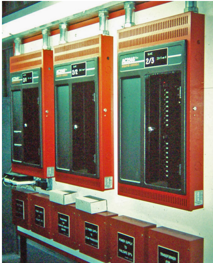
Fig. 3. Direct Digital Control (DDC) panels for air handling units.
