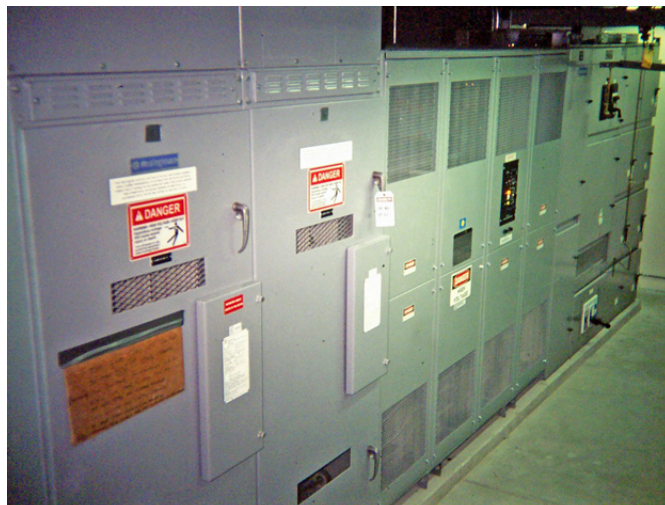
Fig. 1. High voltage electrical distribution system switchgear.
