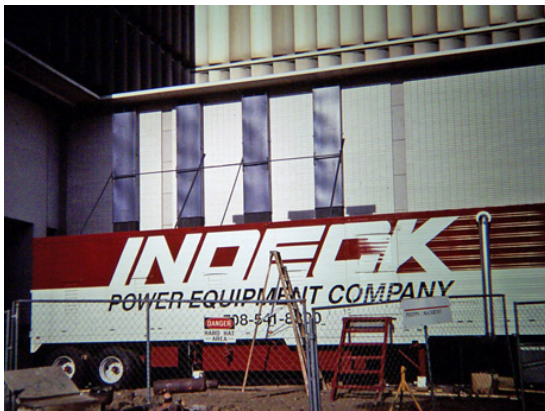
Fig. 7. Truck-mounted steam generator (boiler) to back up existing equipment during construction.
