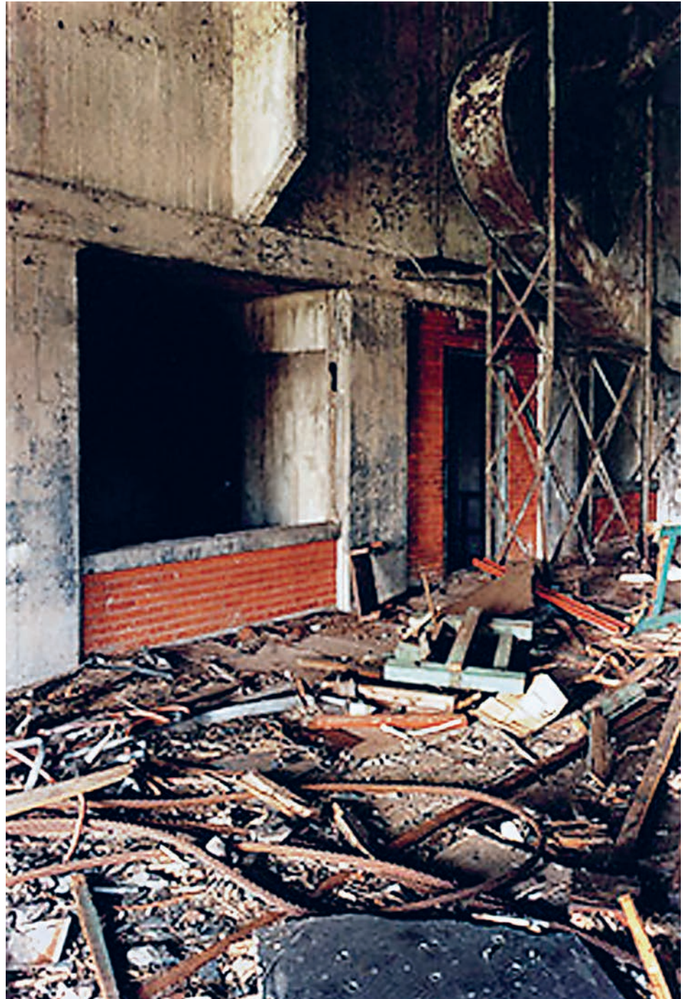
[Fig. 15] Buffalo Grain Elevator. Gerrit Engel. Source: ENGEL, G. Buffalo Grain Elevators . Munich: Walther König, 1997.
