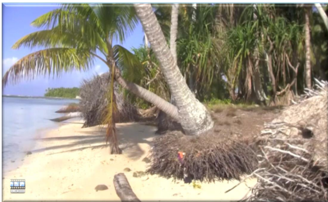
Figure 4 - Coastal erosion on Nukufetau island.
