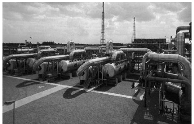
Figure 30. Claus plant for transforming H_2S to elemental sulphur.
