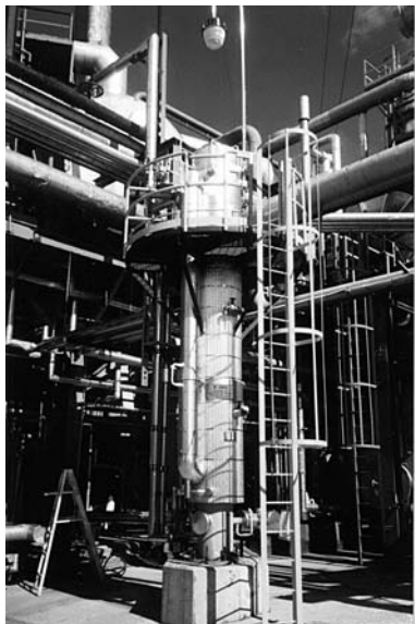
Figure 32. Degasification reactor to accelerate the oxidation of the residual H_2S and polysulfides ( H_2S_x ) to sulphur.
