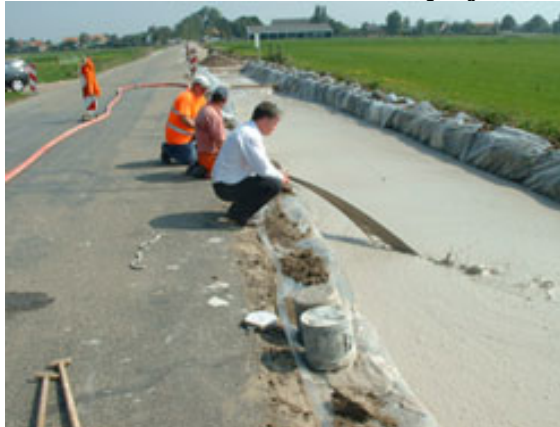
Figure 1: Road in Holland is being widened and foamed concrete was used for the road sub-base
