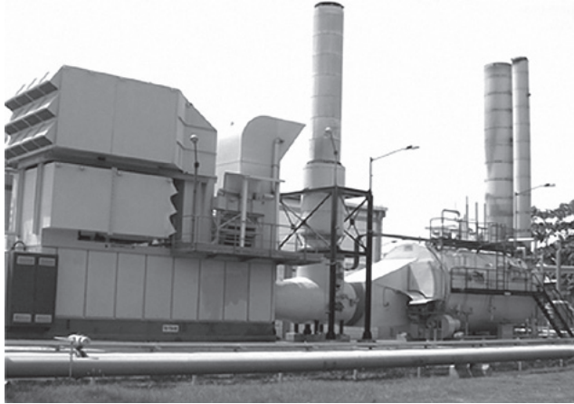
Figure 1. Cogenerator Plant with pirotubular – Shell GT and HRSGs.
