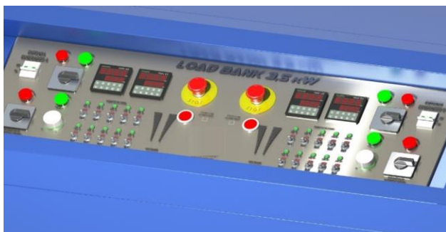
Fig. 11. Main control panel of the load bank.
