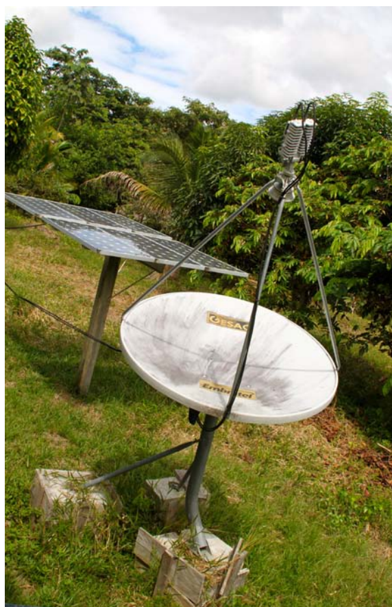
Gesac Antenna and solar panels at Pamáali School
